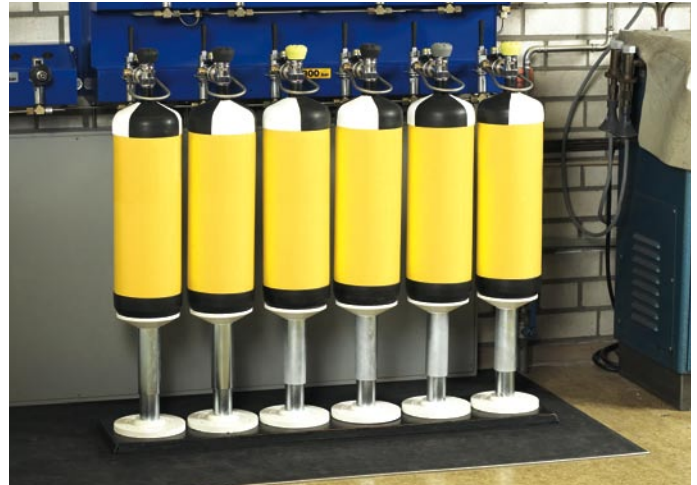
Breathing air adaptors on a filling panel
