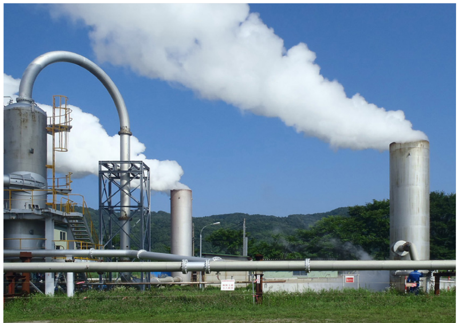
The plumes of steam show that eco-friendly geothermal energy is being produced here.
