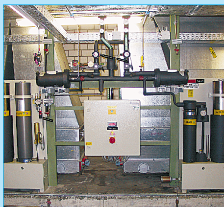
HP-compressor with Seccant IVA dryer activated carbon adsorber, heat exchanger and online dew point hygrometer ■
